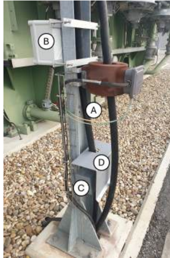
Figure 2: GIC prototype installed at Paraimo substation. A: neutral cable; B: Enclosure I; C: Enclosure II; D: Protection cover.
